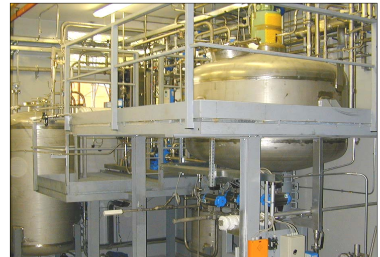
Liquid Effluents Treatment Station
